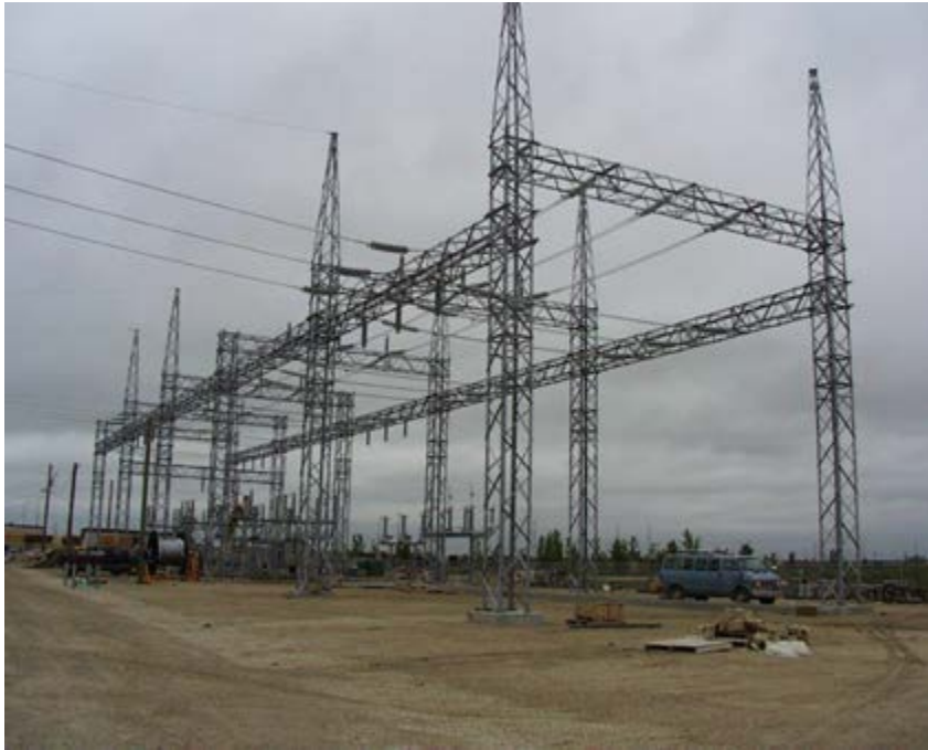
Photo 4-3: Example of steel lattice structures (bus work)
