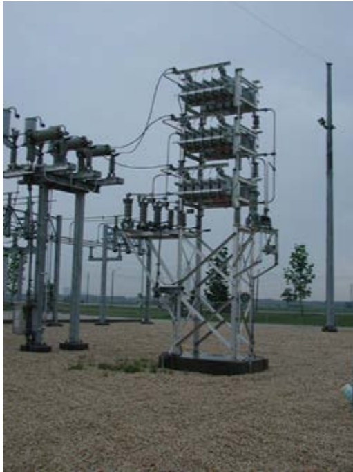
Photo 4-1: Example of manufactured steel supporting structures for a capacitor
