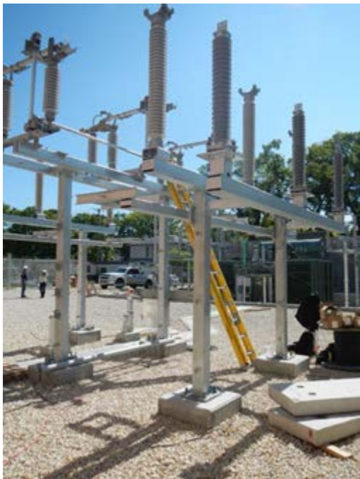
Photo 4-2: Example of tubular steel structures for bus work and related equipment
